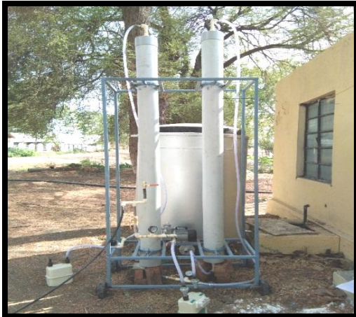
Fig.3 Developed Biogas purification unit
