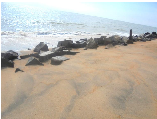
Figure.6 Damaged sea wall at Veliyamcode coast
